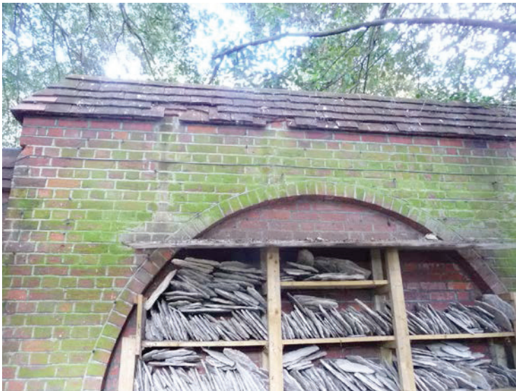
Fig. 6 Boundary wall Access was gained to view the offside of the wall, where many broken tiles were noted. Due to the aspect and covering of vegetation it is possible that bats may use this feature from time to time on a casual basis. The patio garden may be used by nesting birds.
