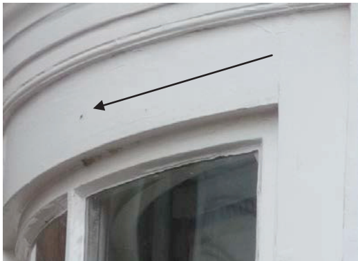
Fig. 2 The arrow marks position of a dropping on the window of the Principals office. Flashing pins above this window were often missing.
