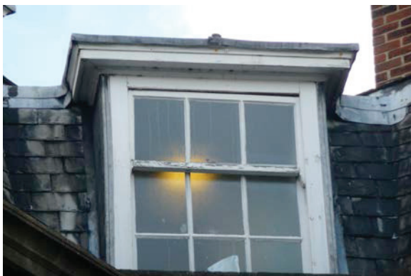
Fig. 3 note deep gaps in flashing on the roofline
