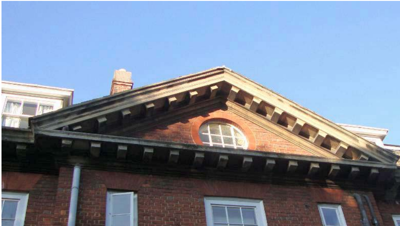
Figure 3: Roof Pediment on internal facade junction between original 1913 Ruskin building and 1930's extension
